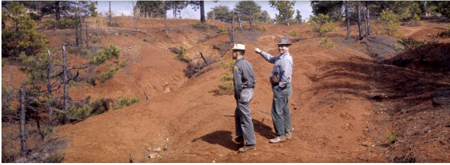
Figure 4. Soil erosion, in this case from poor drainage that caused deep gullies and washed away much of the topsoil, can create difficult growing conditions for trees.
